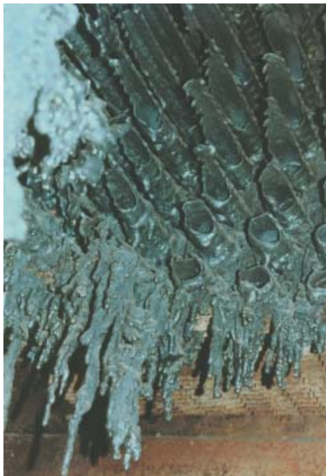
Fig. 16: High temperature fire of a gas fired water tube type boiler
